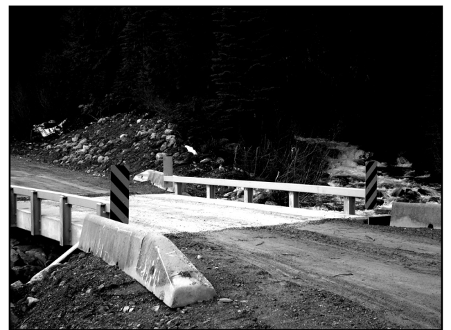
The new cement bridge over the second crossing of the south fork of Gray Creek, installed in October 2009, showing the investment BC Forest Service is putting into maintaining the road.
