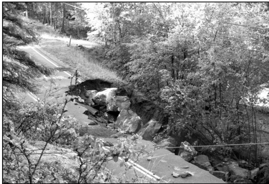
Washout of Highway 3A in Gray Creek
