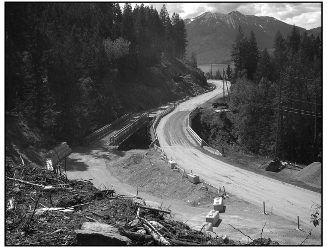
The Bailey Bridge at the Akokli Creek/Cummings Corner is operational. The traffic light wasn't ready when the photo was taken. One worker said that they will be there until November. We don't think there will be much delay with a traffic light system – Boswell's first. What's missing? Arnold Cummings to supervise!
