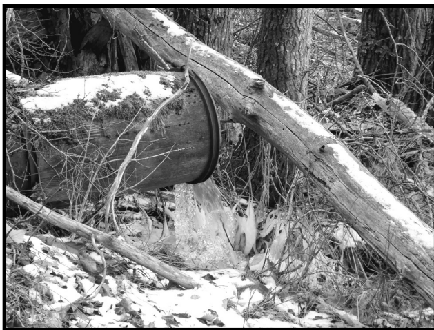
Oliver Creek crosses under Hwy 3A in this 1946-era wooden culvert, coming out between the 7th and 8th tree in the row of plane trees (counting from the north), and flows into the lake. Cooped with staves like a barrel, the culvert is still watertight 75 years later. Photo and discoverer: Janet Schwieger, Feb. 16, 2021
