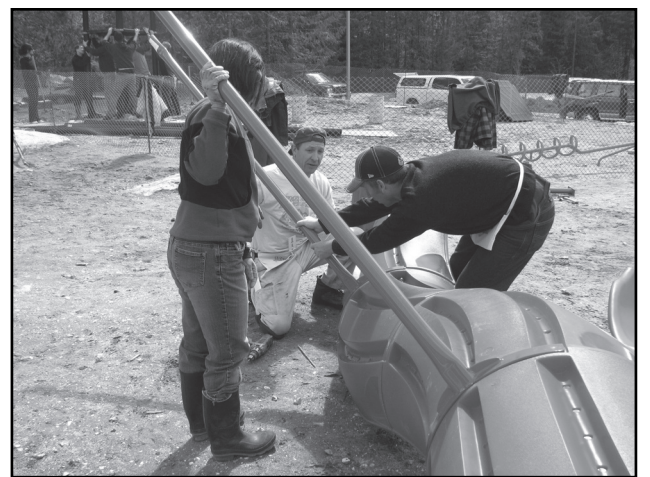
Photos from playground installation day at CBESS, April 24. Top: Serge Darchen, Kevin McBride, Dano Cheverie and Sal Couling lift the first platform of the fort structure. Middle: the auger digs holes for the swing set. Bottom: Dana Gallinger, Dave Ring and Juergen Baetzel assemble the slide. Photos Ingrid Baetzel
