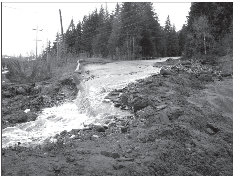
Shown here: the bottom of the south end of Crawford Creek Road with heavy water/mud run-off closing it off to traffic due to a mud slide on the night of April 26.
