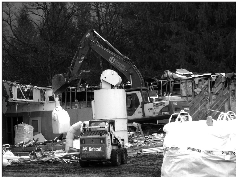
Demolition of the old Crawford Bay School is in progress. Large white bags containing asbestos and possibly other material are being moved by machine to a demarcated area at right for special disposal.
