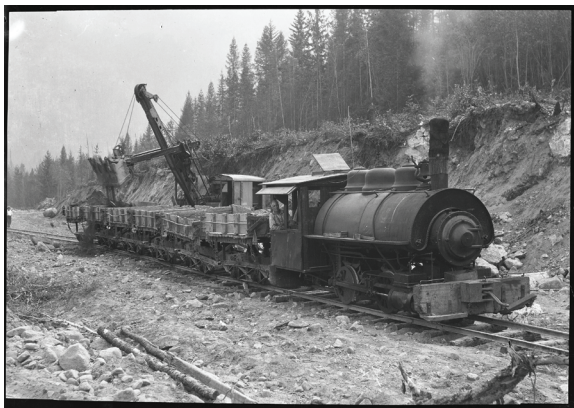
The little No. 30 steam locomotive at work on the new CPR line between Kootenay Landing and Procter, 1929-30. It was built in 1913 by the Porter Steam Locomotive Works, Pittsburgh, PA. Photo: Nelson Museum, Archives & Gallery.
