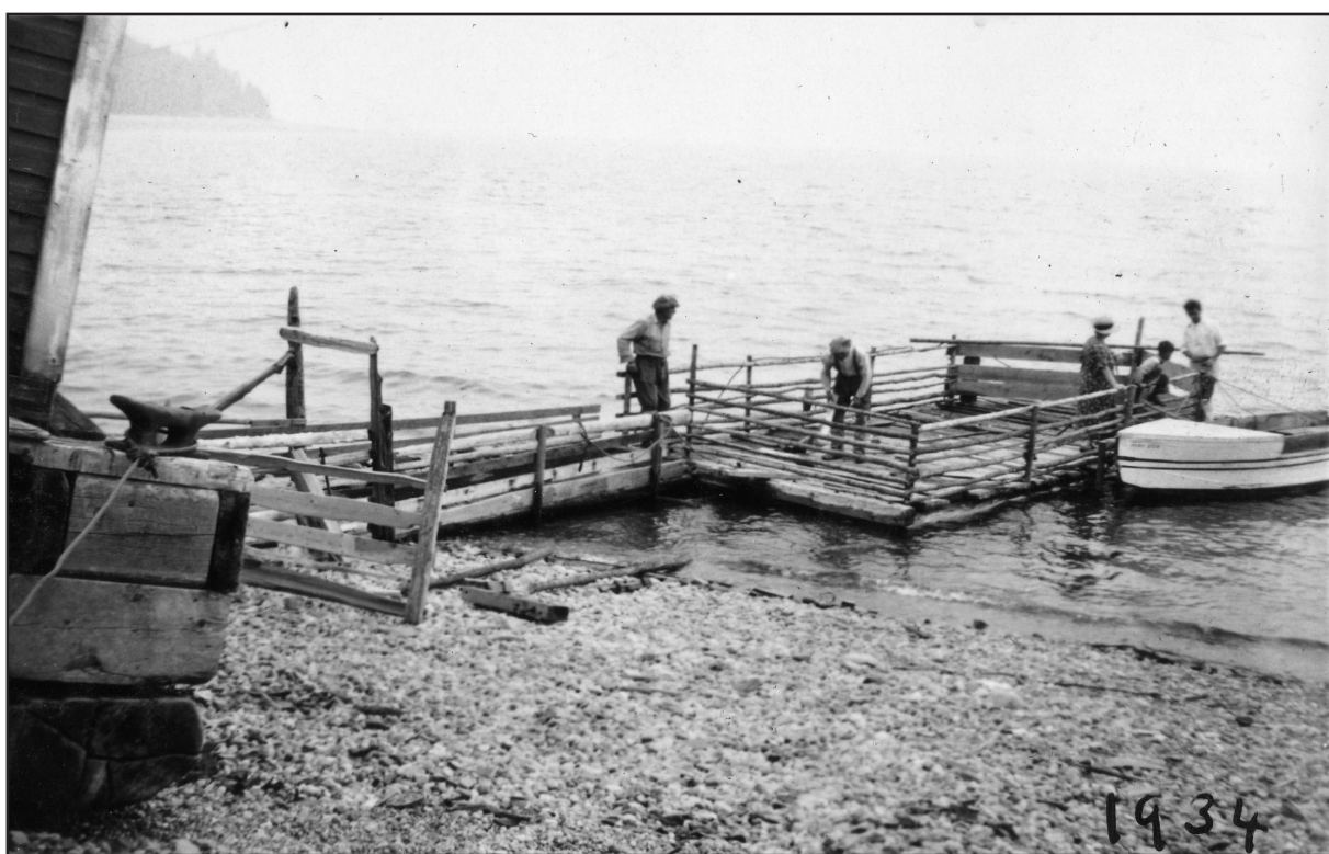
Above: Building the floating sheep pen at Walker's Landing south of Riondel, 1934. From Graham Brown album via Brenda Dau
